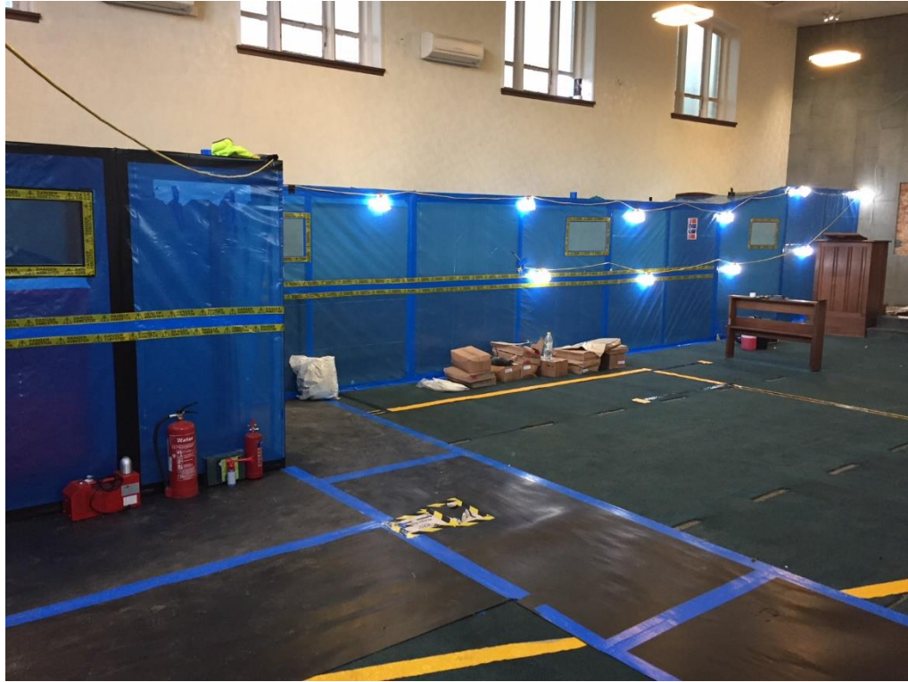
Photo 6: Preparation for removal of concealed asbestos
